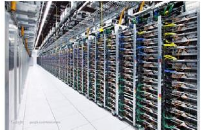
Racks of servers (and switches at the top), at Google's Mayes County, Oklahoma data center [extremetech.com]
