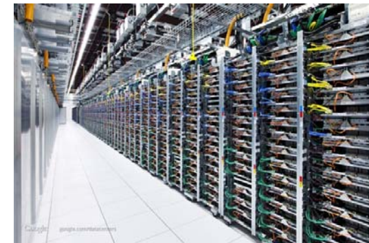
Racks of servers (and switches at the top), at Google's Mayes County, Oklahoma data center [extremetech.com]
